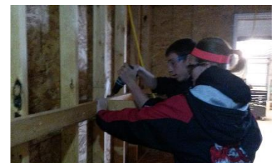
Nikki Schmidt and Dylan Sexton work to finish off a garage to be used for storage.
